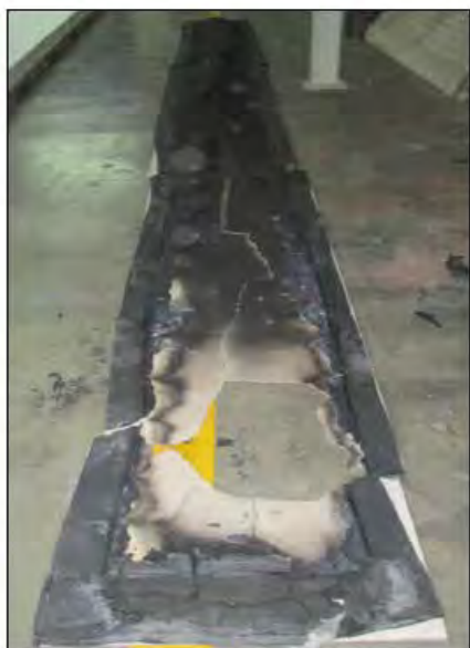
Photo 3: Specimen after the test (located near the fire end)
